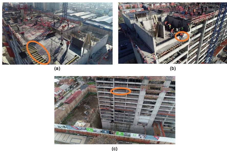
Figure 3. UAV images for safety monitoring at a construction site in Chile: (a) lack of guardrails; (b) worker without safety rope; and (c) lack of guardrails (Images by Jhonatan G. Martinez) [23].
