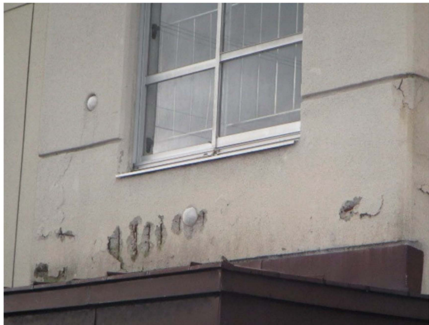
Figure 4. Spalling of concrete due to cracking and corrosion in a cold climate [24].
