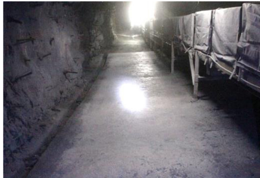
Figure 6. Deformation control effect of lane 1105.
