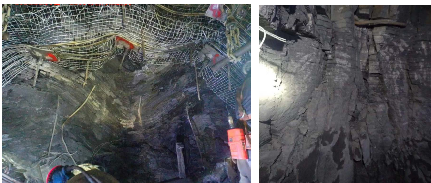
Figure 2. Deformation and failure characteristics of surrounding rock.
