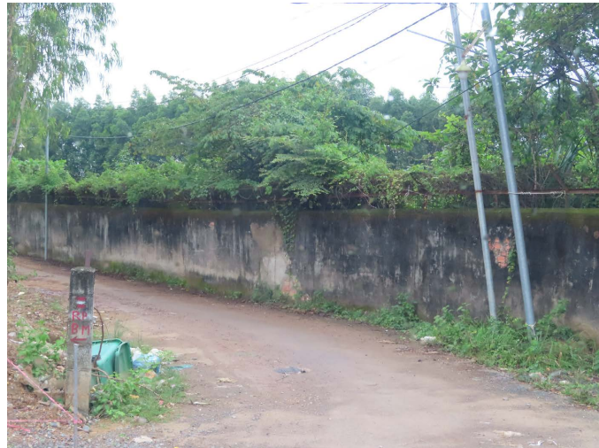
Figure 25. A cement perimeter fence at the Bien Hoa Air Force base. The jungle vegetation was similar to the vegetation surrounding all the Vietnam Air Force bases in the 1960s, were sprayed with tactical herbicides.
