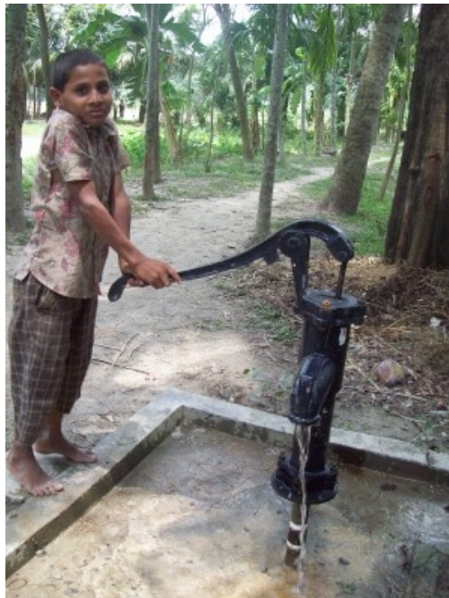
Figure 9. Tube wells in the Mekong Delta. Reprinted with the permission of the editor of the Open Journal of Soil Science.
