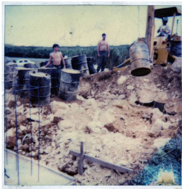
Figure 30. Re-packing herbicide barrels and recovering buried barrels leaking into the ground. Reprinted with the permission of the editor of the Open Journal of Soil Science.
