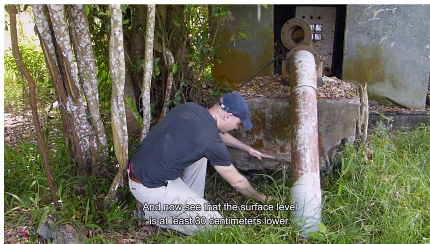
Figure 12. Approximately 30 cm of subsidence around a pump station structure in Jakarta. Credit Line: Courtesy of the Jakarta Post.
