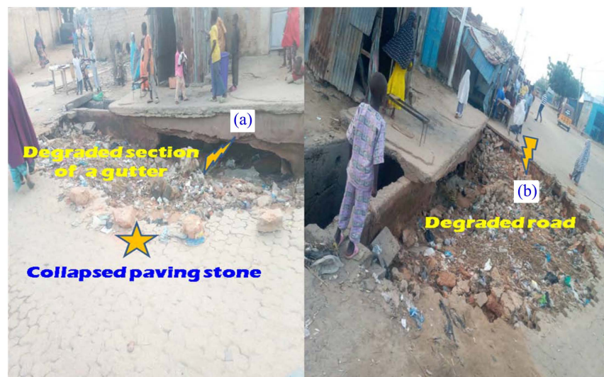
Figure 9. Views of a damaged canal (a) and a degraded road (b).
