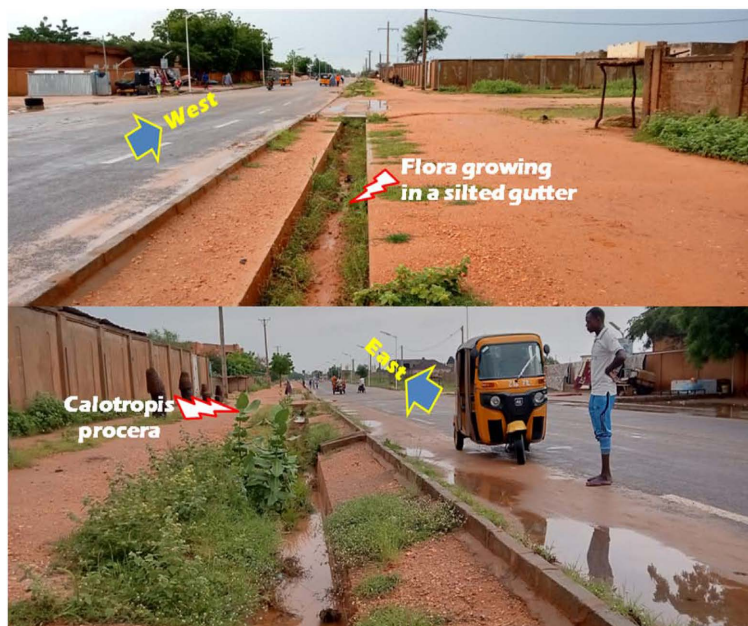
Figure 7. New gutter in the Ali Dan Sofo District subject to silting and the establishment of diverse flora and vegetation during the rainy season. Source: field August 2023.
