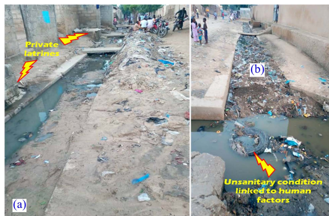
Figure 5. Status of rainwater harvesting facilities in the municipality II, according to the reality of the ground. (a) Old gutter connected to private latrines. (b) Old gutter considered as a receptacle for all types of waste.
