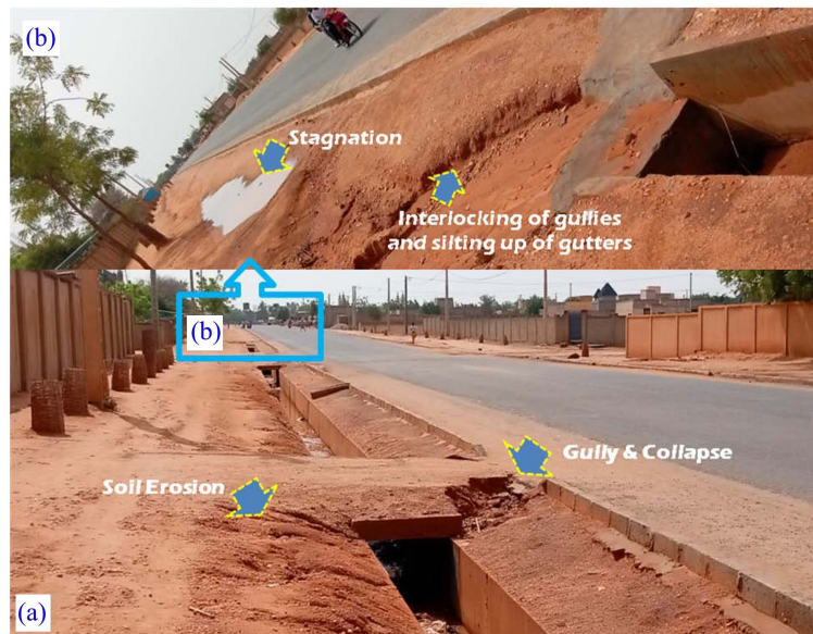
Figure 6. Runoff, erosion and gully (A) around the new gutters of Ali Dan Sofo (Commune III of Maradi). Insert (B) highlights the processes of rainwater gully along roadways and upstream of structures. Source: fieldwork 2022.
