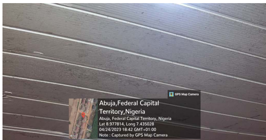
Plate 5. Polyvinyl chloride (PVC) ceiling used in Sunrise Estate. Source: Field Work, 2023.
