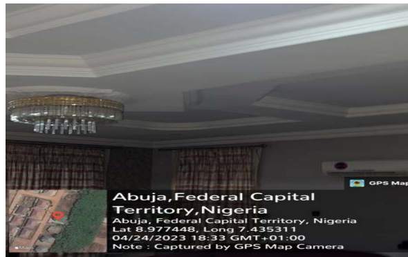
Plate 6. Plaster of Paris (P.o.P) ceiling used in Efab Estate. Source: Field Work, 2023.
