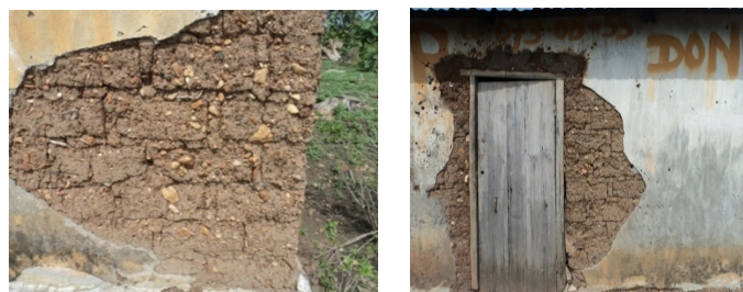
Figure 3. Peeling of the body of the coating.
