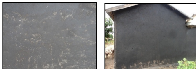
Figure 2. Leaching of the surface layer in bitumen.
