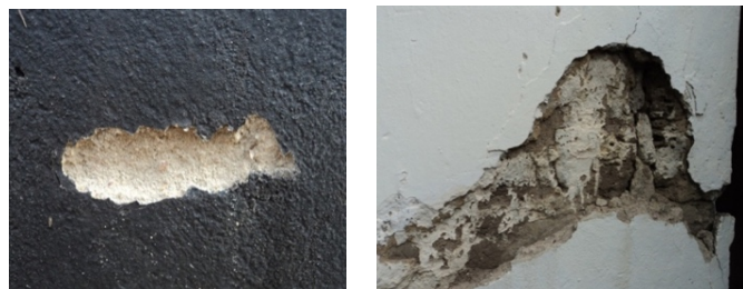
Figure 1. Crumble of the coating.
