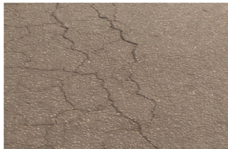
Figure 6. Pavement cracks due to temperature and traffic pressure.
