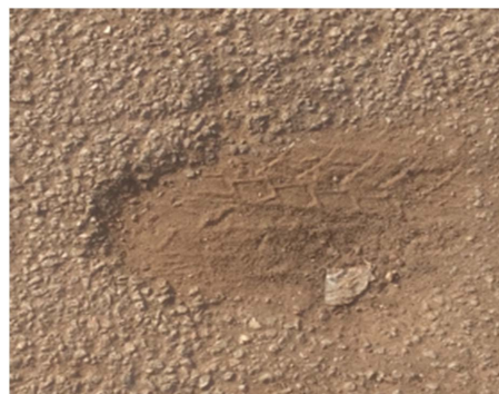
Figure 7. Potholes due to traffic pressure.
