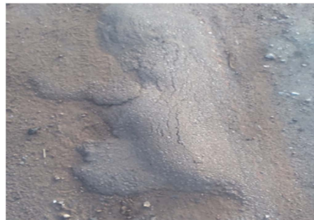
Figure 5. Pavement deformation due to temperature and traffic pressure.
