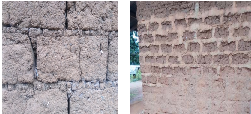
Figure 3. Erosion and cracking of unstabilised mud-brick walls exposed to rain. West Cameroon.
