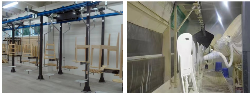
Figure 4. Robotic system with hanging conveyor belt.
