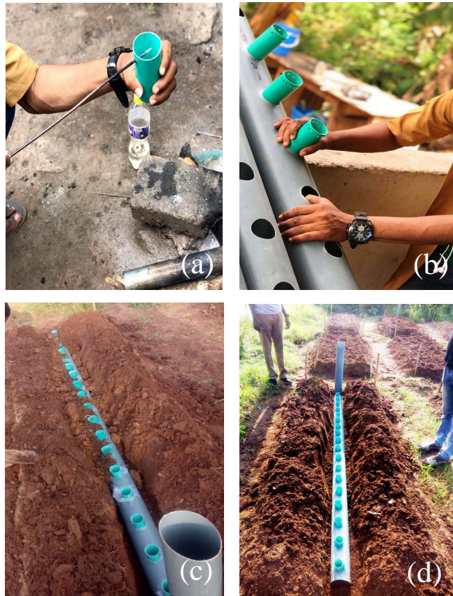
Figure 2. (a) Making of 3 - 4 mm holes round one end of each of the capillary pipes, (b) Fixing of the capillary pipes into the holes on 10 cm diameter pipes, (c) Installation of the constructed irrigation system, (d) Complete Sub-surface irrigation system on the experimental plot.
