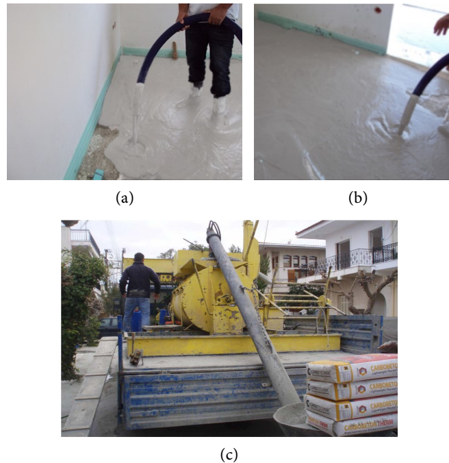
Figure 1. (a) and (b) application of the newly developed screed on 5 m 2 floor. (c) the screw-type pump used for the test.
