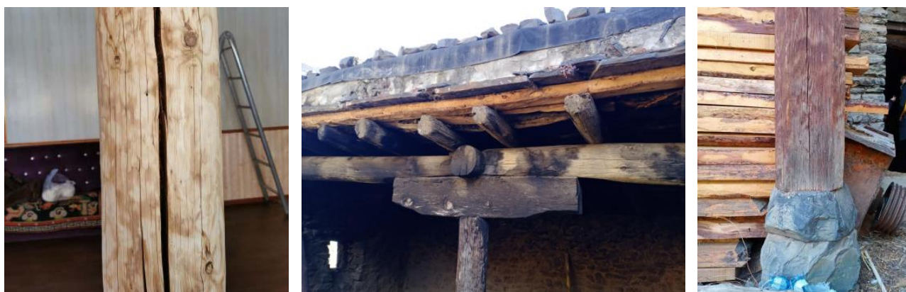
Figure 2. Damage condition of wooden structure of residential houses (Photo source: taken by the author).
