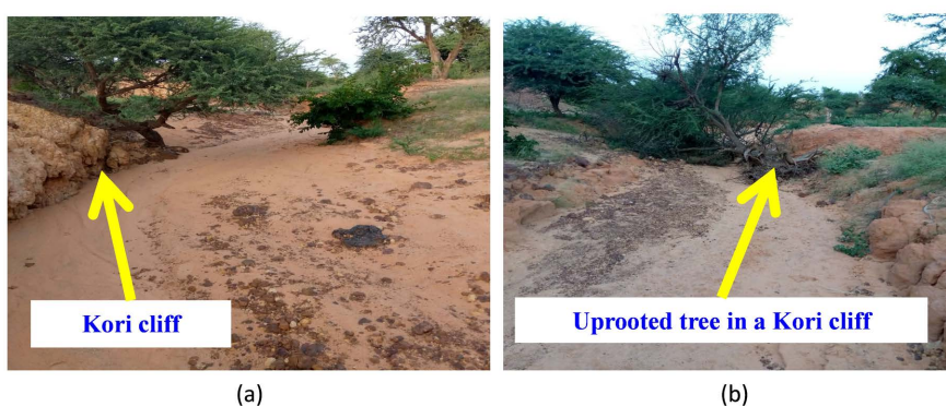
Figure 11. Consequences on the slopes of the influence of the new morphodynamics in the current landscape.
