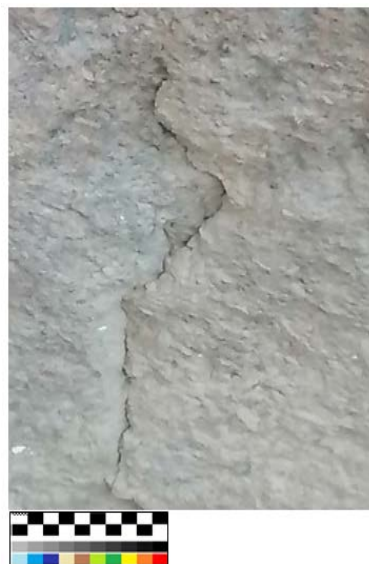
Figure 16. Weakness, fragility, fragmentation and cracks.
