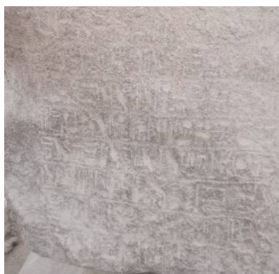
Figure 5. Corrosion, loss, gaps, and Peel off the text hieroglyphic.
