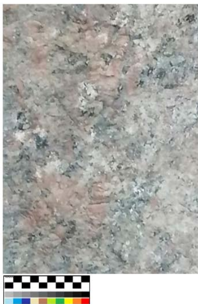
Figure 15. Erosion and peeling of the surface layers.
