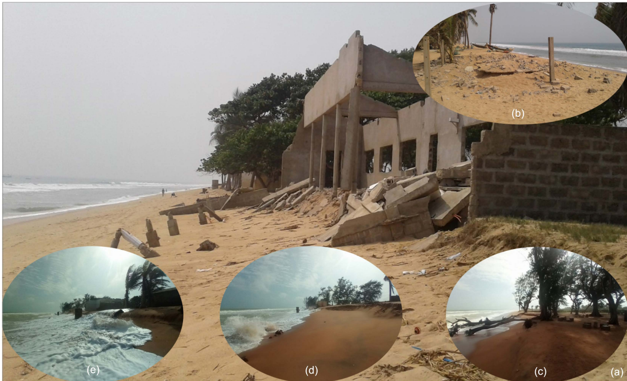
Photographic Plate 2. Littoral sud-ouest du Bénin: Views of damage caused by coastal erosion in the commune of Grand Popo 2021-2022. (a) Buildings of the Christian celestial church completely in ruins (Ayiguinnou) (b) Destroyed houses in Hilacondji (c) Completely destroyed rest area in the filaos district of Agoué (d) Completely eroded shoreline in Agoué (e) Houses damaged by coastal erosion in Kindjèhoué beach).
