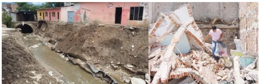
Figure 5. UCA and house, collapsed [19].
