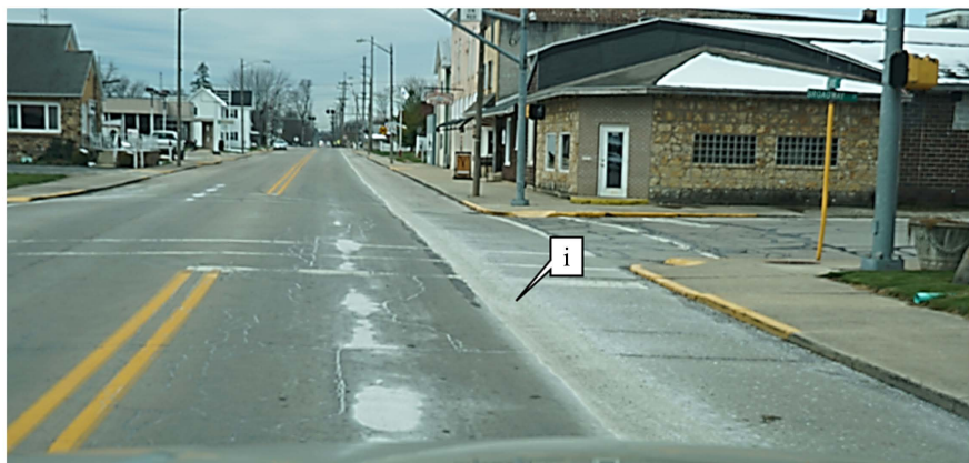
Figure 3. Salt residue from over-applied salt.
