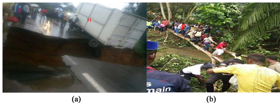
Figure 8. A section of road collapsed and passengers crossing on foot. (a) Collapse of a culvert along the Douala-Yaounde National Road Note the van trapped and stranded passengers observing the scene (Source: Nnecdem, 2019); (b) stranded passengers crossing a bridge with the help of security agents to get relay buses for their journey (Source: Ojuku, 2019).
