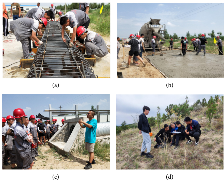
Figure 1. Practice training site. (a) Binding main beam reinforcement; (b) Prefab site construction; (c) Field lectures by experts; (d) Field line selection & measurement.
