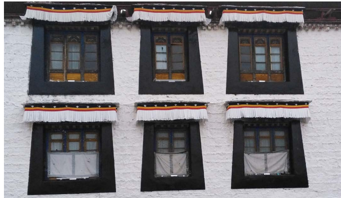
Figure 2. Detail of window of Potala Palace (the source of the photo: self taken by the author).
