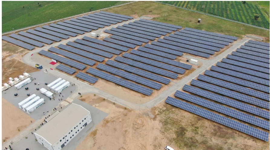
Figure 4. A solar hybrid power plant.
