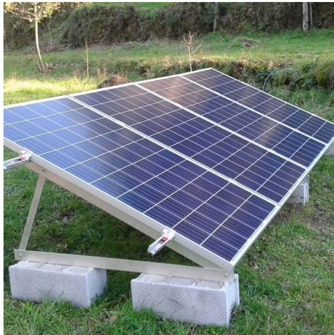
Figure 6. Standard solar panels.
