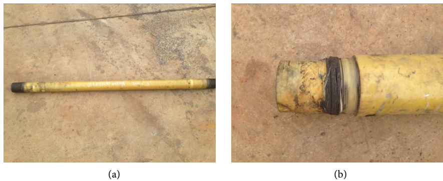
Figure 2. Short time water pressure failure morphology. (a) Pipe leakage; (b) Joint thread debonding failure.
