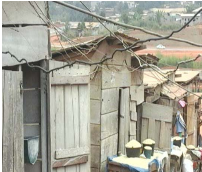
Figure 7. Market stores (warehouses). Notice the poor building materials and the passing of electrical cables.
