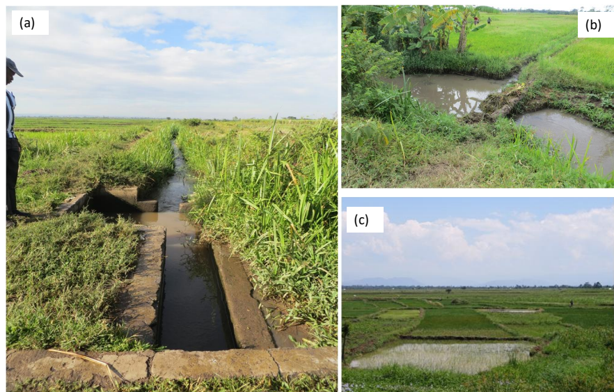
Figure 3. (a) Dilapidated canal and division box; (b) Locally made diversion; and (c) Rice at different growth stages.
