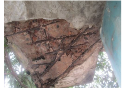
Plate IV: Concrete spalling observed on second floor slab.
