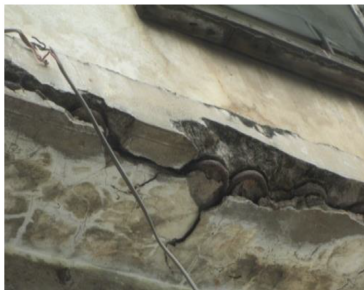
Plate III: Concrete spalling on first floor slab.
