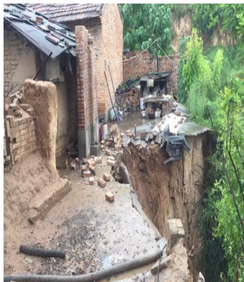
Figure 4. Image of the landslide behind the white building in the building materials factory.
