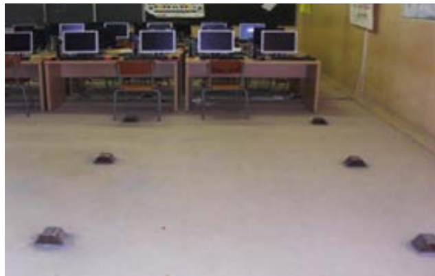
Figure 2. Electric sockets mounted on the floor of the computer Labouratory.
