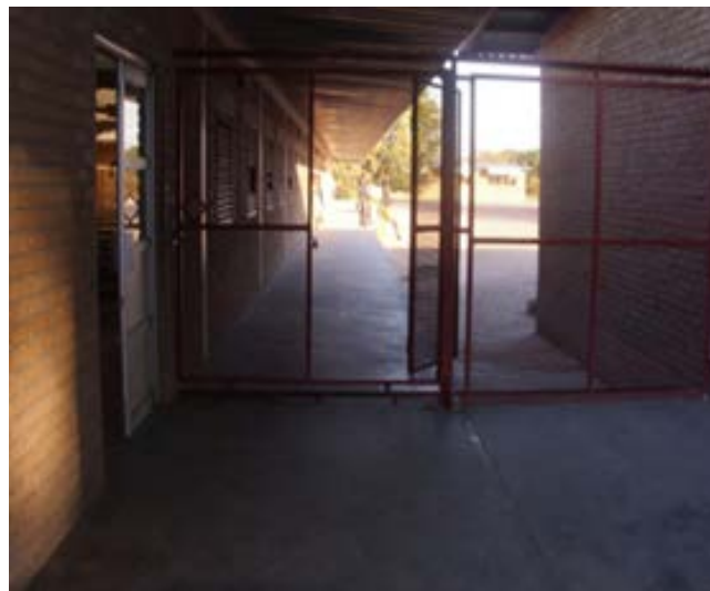
Figure 3. High corridor pavements and obstacles.
