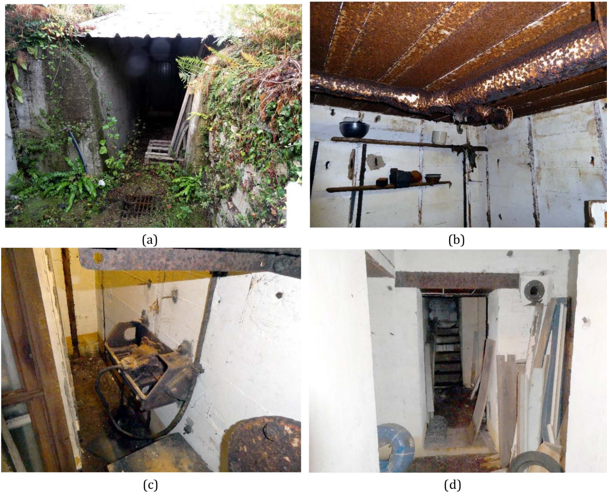
Figure 2. R 628 (12): (a) Entrance; (b) Crew room with supports for reclining cots, rusted ceiling and aeration conduits; (c) Support for telephonic connections; (d) Exit stair.
