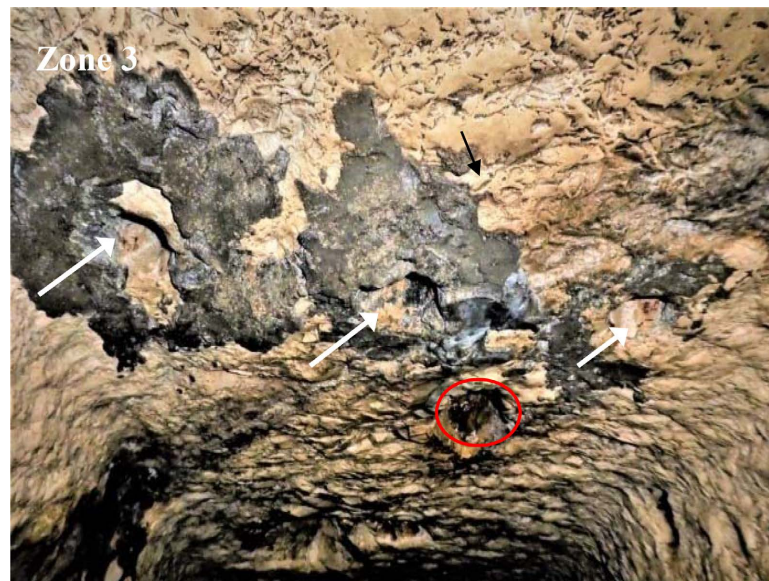
Figure 16. Tunnel ceiling, alteration Zone 3. Three hand-carved depressions (arrows) roughly encircled with a layer of black pozzolanic mortar. Another depression with a rust interior is present beneath (encircled red). (see Table 2 , Table 3 , Analyses for Zone 3).
