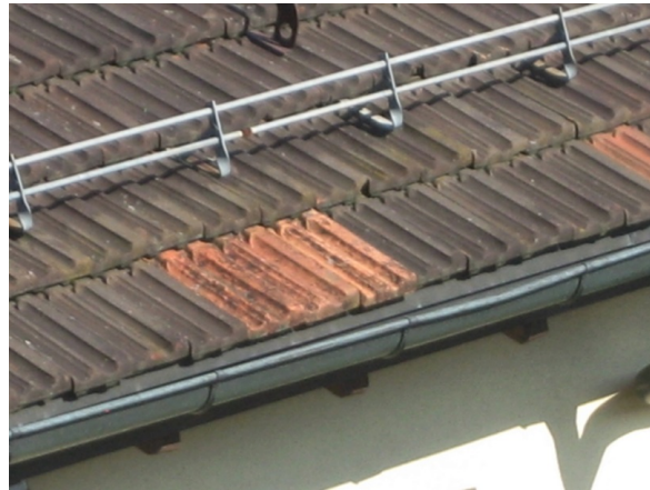
Figure 22. Aged roof with some recently replaced bricks.
