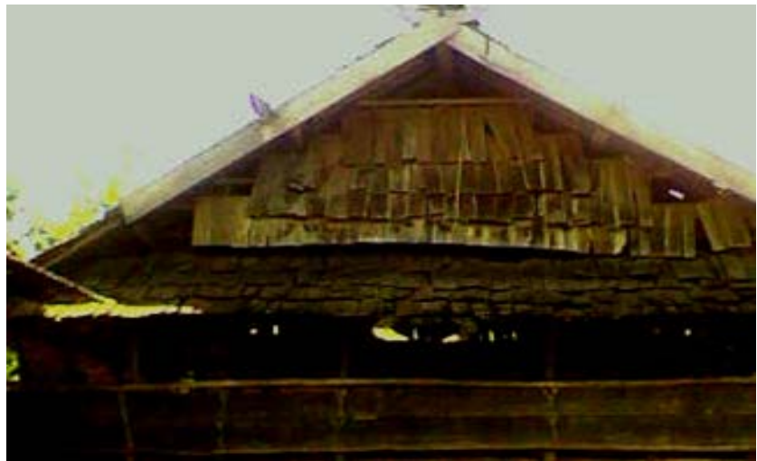
Figure 13. An example of utilizing bamboo as a roof. Source: Researchers' recorded images in 2010.
