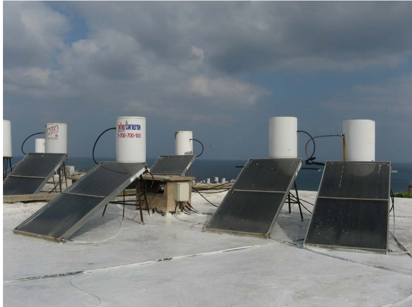
Figure 11. The water-boiling tanks consist of a so-called mirror, which is a cage covered with translucent plastic, inside of which are a number of copper tubes that lead the water to the collecting tank. Photograph by the author.
