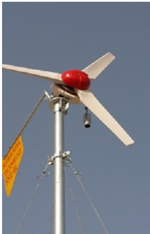
Figure 10. 0.7 kW SNT-1 rooftop wind turbine installed at GERMI rooftop.
