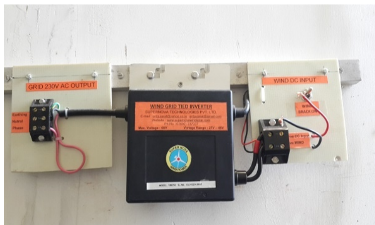
Figure 11. Grid tied inverter for SNT-1 wind turbine.
