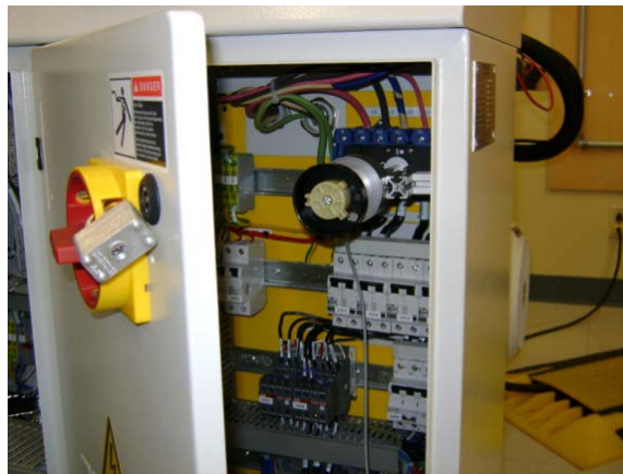
Figure 7. Rotary potentiometer installed on the electrical panel.
