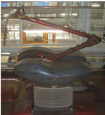
Figure 1. Photograph of the pantograph.
