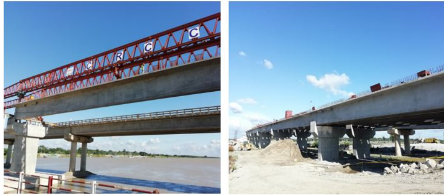
Figure 3. Launching of T-Girder on Temporary Bearing at Arial Kha Bridge, Shibchar, Madaripur, Dhaka, Bangladesh.
