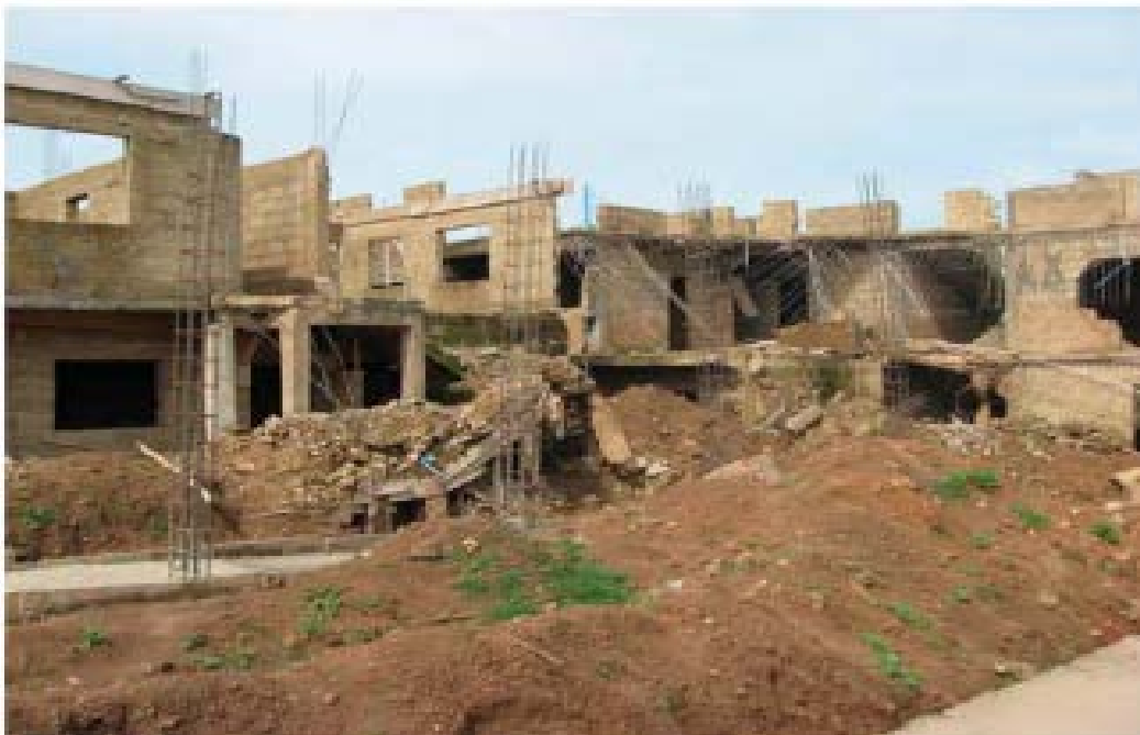
Figure 1. Collapsed part of the building.
