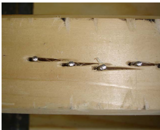
Figure 5. 7d nail spacing cracks.
