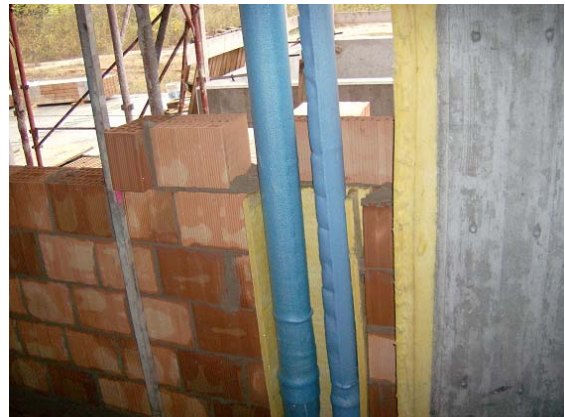
Figure 6. Thermal and acoustic bridge avoiding using proper plumbing sheath and fibrous material.
