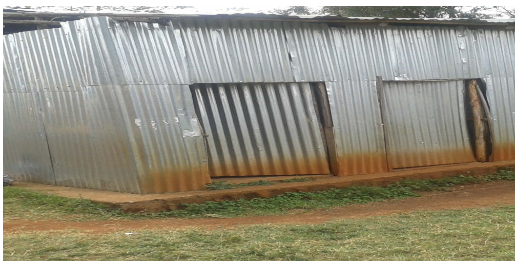
Photograph 3. Dilla university community KG School toilet (February 2014).
