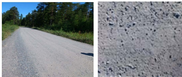
Figure 2. The unpaved road in Hertsö and the road surface.
