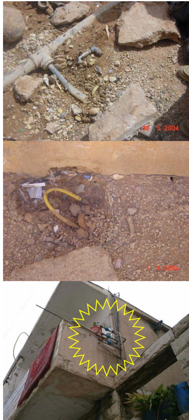
Figure 8. Examples of administrative loss in Mafraq: up—the meter is removed and replaced by a T-joint; middle—pipe connection passing the meter; down—connection to supply the housing unit before the meter.
