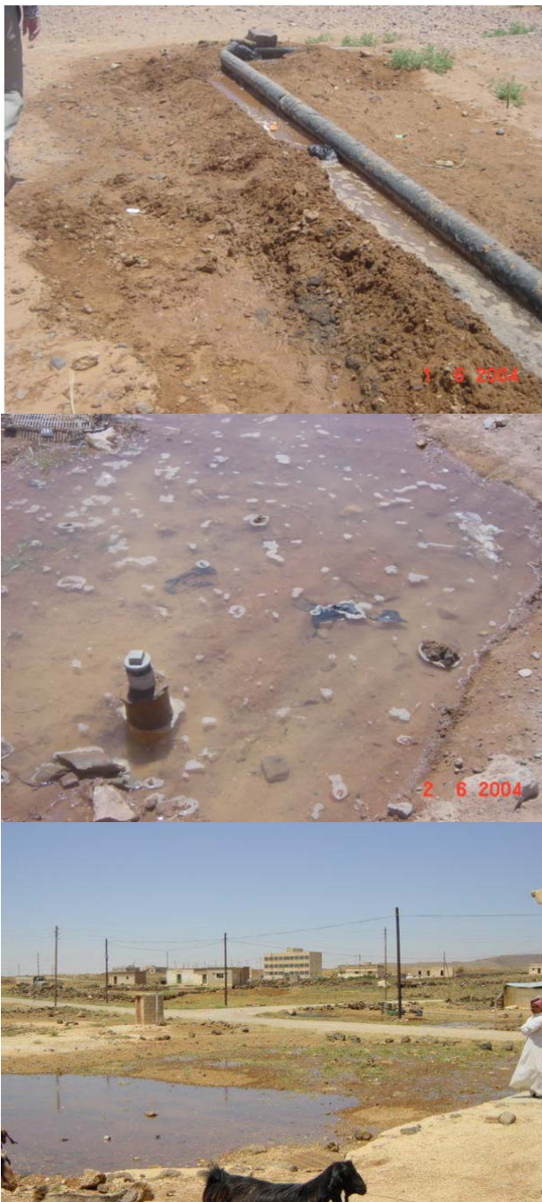
Figure 7. Examples of technical losses: up—broken pipe; middle—leaking pipe; down—breaking pipe to supply water to livestock.
