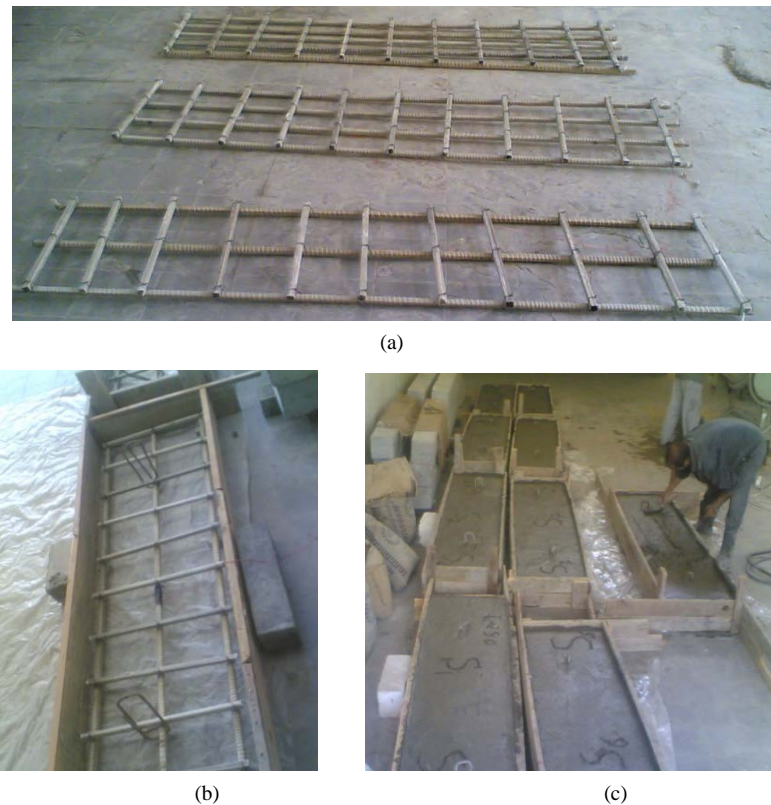
Figure 4. Fabrication process of the slab specimens: (a) Overview of the of the assembled GFRP cages; (b) GFRP cage inside the formwork; (c) Slab specimens after casting.
