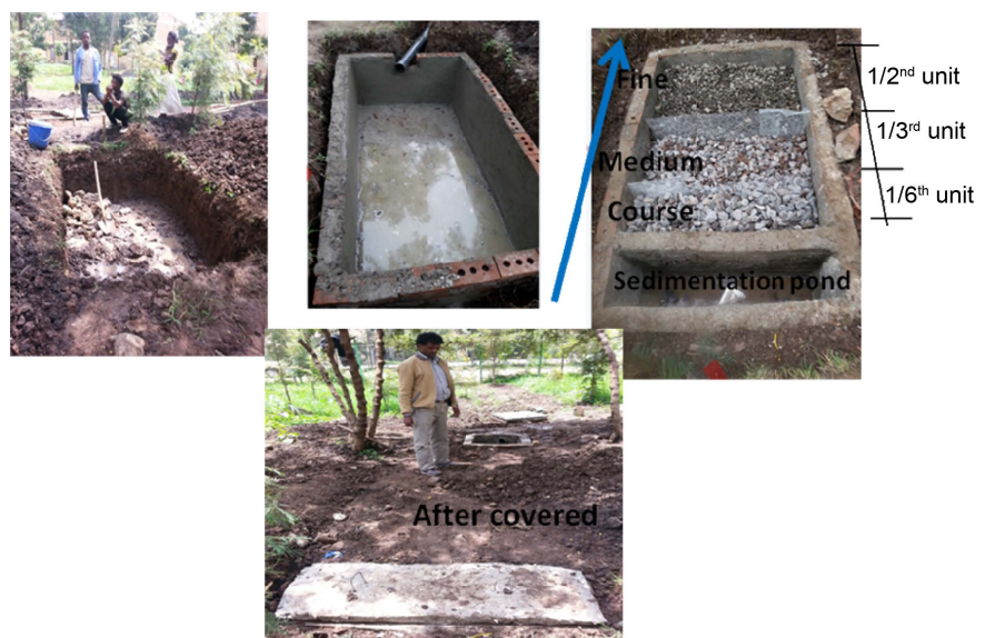
Figure 4. The low-cost stormwater filtration system from excavation to filling the system with filtration media (top) to making the system ready for performance test (bottom).
