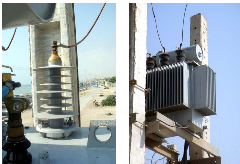
Figure 6. Sample bushing installed in the network.
