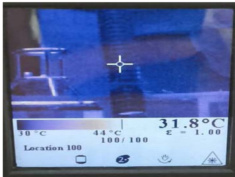
Figure 4. Temperature of arrester with 12.8 kVrms ac voltages applied and ESDD at 0.285 mg/cm 2 .
