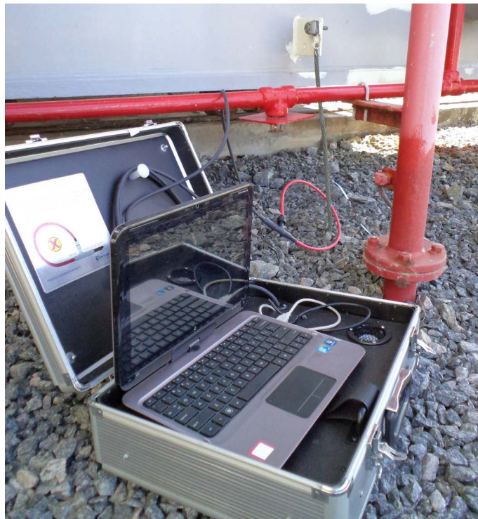
Figure 12. Installation of the proposed device in the grounding of the 29 MVA transformer.
