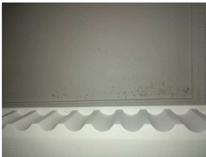
Figure 3. Mould under the ceiling in newly completed building.
